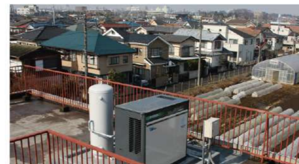
Component manufacturing plant: SMS11ED x 1
