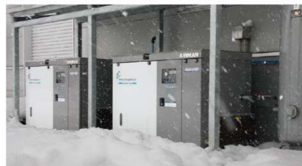
Manufacturing plant: SMS15SD x 2
